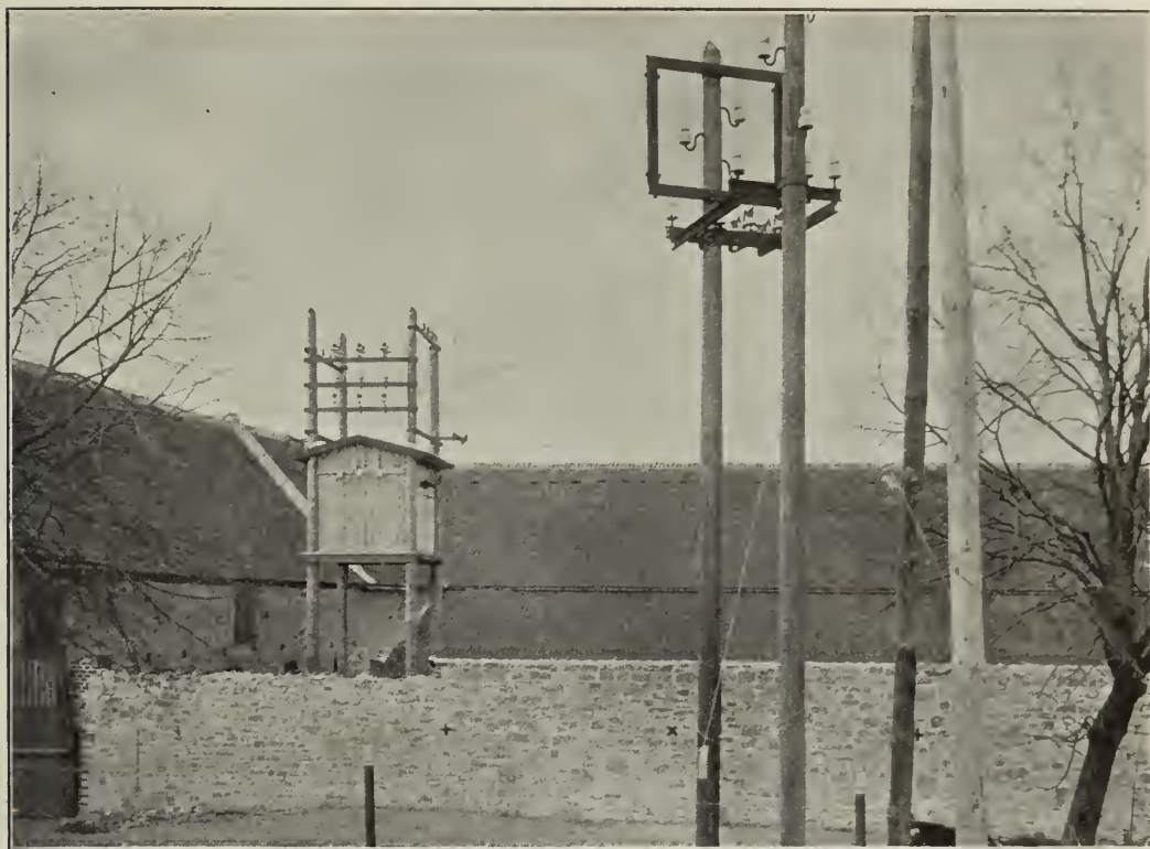
TRANSFORMER HOUSE RAISED ON POLES, CROTTORF.
